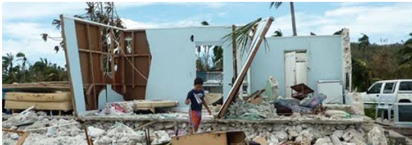
Cyclone damage to housing — the kind of immediate impact this recommendation responds to.
